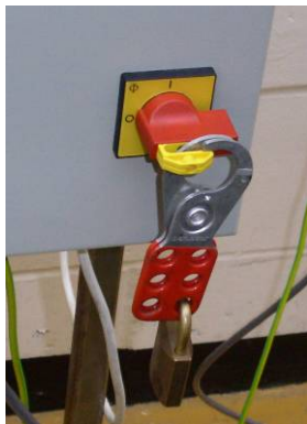
Figure 7-1 Panel with power 'locked off'
